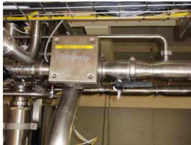
MA-700 In-pipe analyser on condensed milk line
